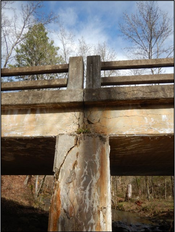
Advanced Deterioration on Center Bridge Pier
