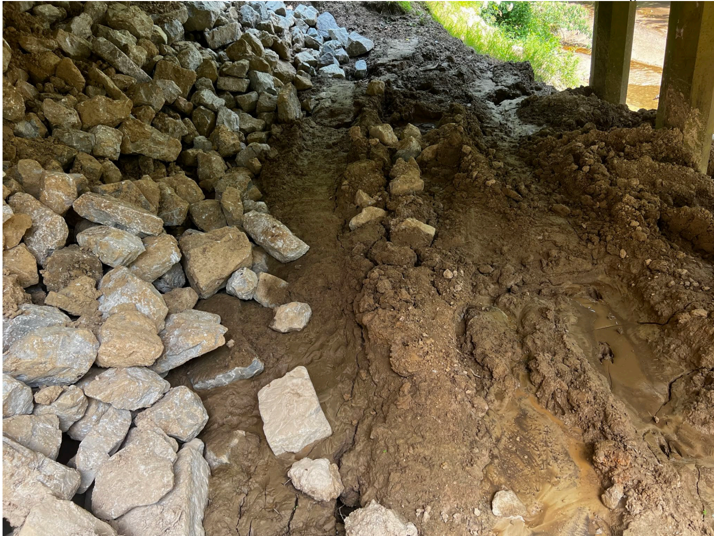
Site 2-Locust Creek another view of failed soil under south abutment
