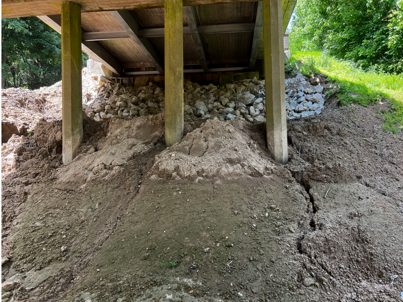
Site 2-Locust Creek slide at the south abutment in silty clay
