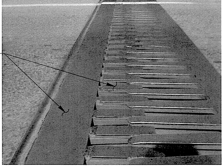
PHOTOGRAPH OF FINGER JOINT TO BE REPAIRED
