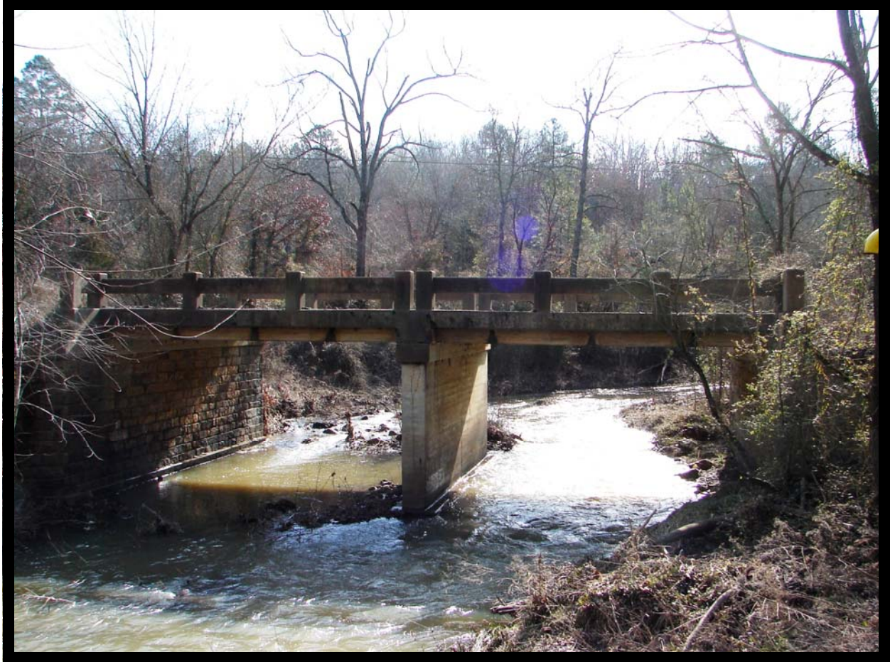
EVALUATION BRIDGE #14791 SHAVER ROAD (Co. Rd. 49) LOGAN COUNTY CONCRETE CONTINUOUS SLAB DATE OF CONSTRUCTION – 1942 BUILDER - WORKS PROGRESS ADMINISTRATION
