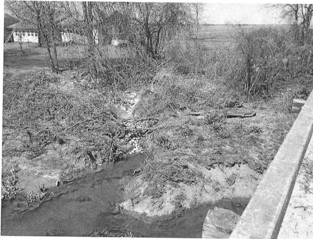
Figure 3. Scouring in drainage on the up-station side of the channel and west side of the roadway.
