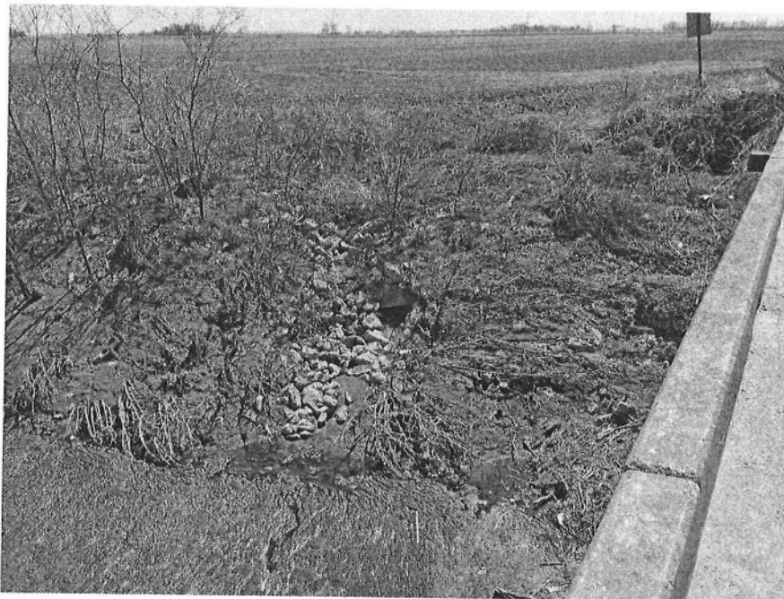
Figure 2. Scouring in drainage on the down-station side of the channel and east side of the roadway.
